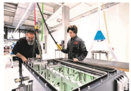
Endmontage eines Energy Storage Systems (ESS)
